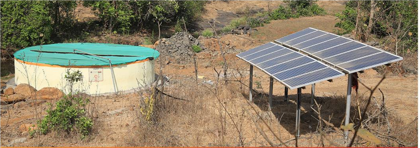
Water source in Zorewadi and solar panels used for lifting water to storage reservoir
